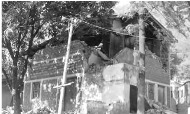
Figure 7.1 : A Damaged Building Due to an Earthquake
